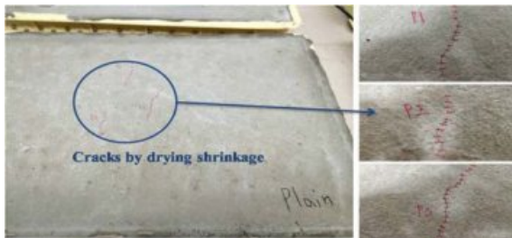
Fig. 2. Cracks that formed due to drying shrinkage.
