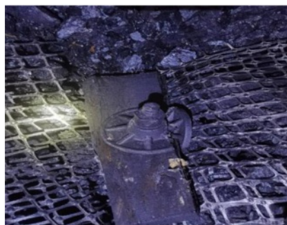
(a) The crack of the edge
