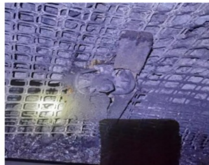
(b) The crack of the center
