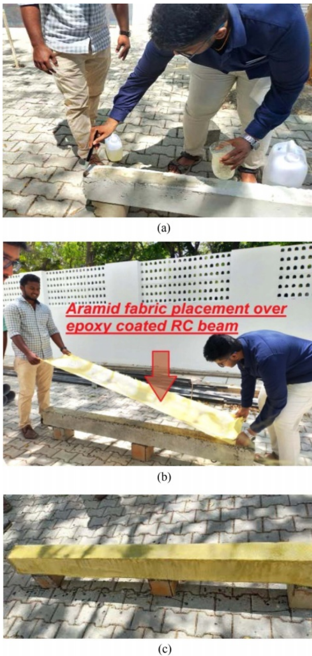
Fig. 5. (a) Application of Epoxy over RC Beam Specimen. (b) Placement of aramid fiber matrix over epoxy coated RC beam specimen. (c) Aramid fiber reinforced RC beam.
